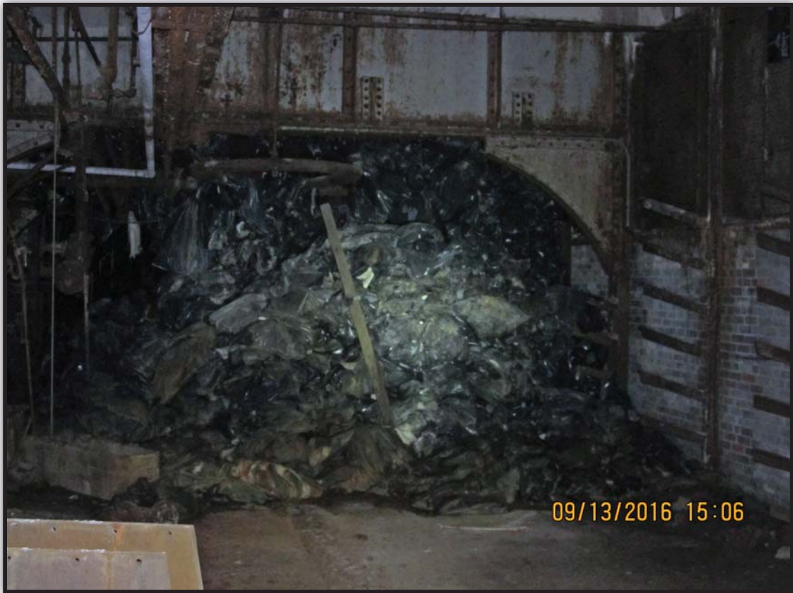
PHOTO 3. English Station - First Floor, west side of low pressure boiler
