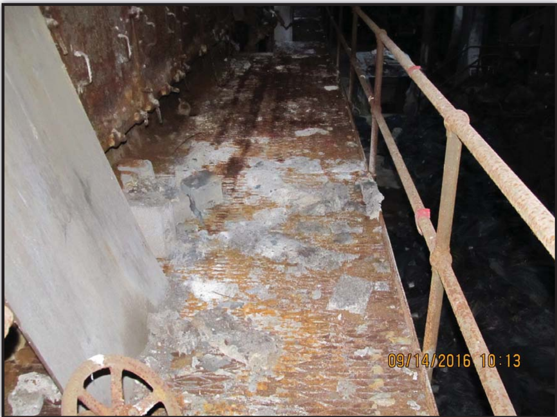
PHOTO 2. English Station - low pressure boiler area.
