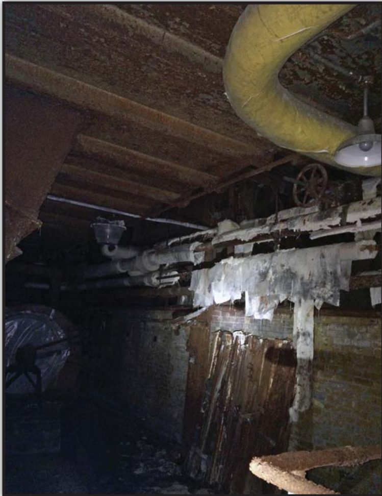
PHOTO 6. English Station - First Floor, west side of low pressure boiler area.
