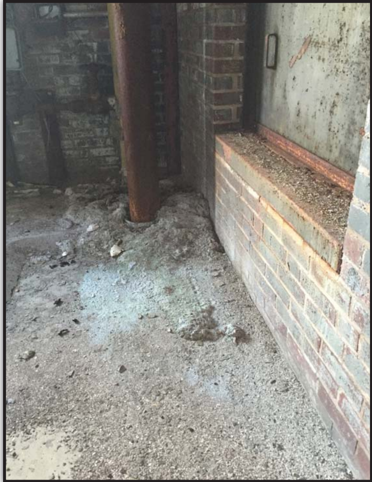
PHOTO 5. English Station - First Floor, east side, vicinity of Lighting Panel "OR."
