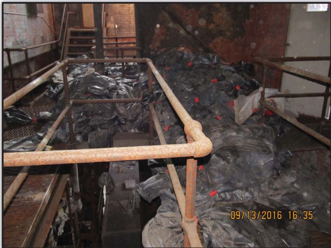
PHOTO 4. English Station - north end of low pressure boiler area.
